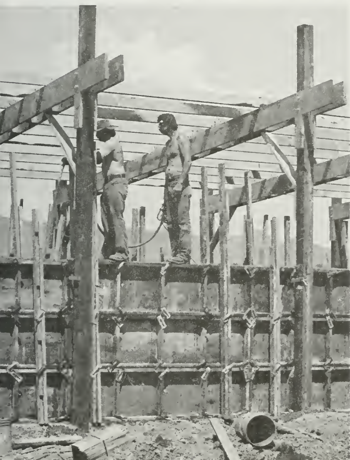
Construction jobs were yet another benefit of the Rural Clean Water Program in Tillamook County. Here, carpenters build a dry manure storage structure that will have a roof to deflect the high annual rainfall in the area.
